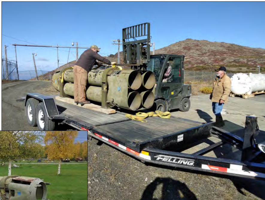
Gordy Heinen checks the contact between the forklift tines and the loading straps before the booster is lifted off his trailer at Site Summit. Lance Morgan, right, supervises. (Photo by Doris Thomas)
